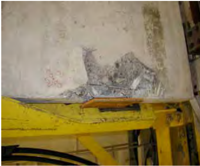
Fig. (12b). Concrete slab damage sustained as a result of testing Connector C in horizontal reversed cyclic shear.
