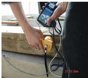
(a) Measure of cracking width caused by corrosion
