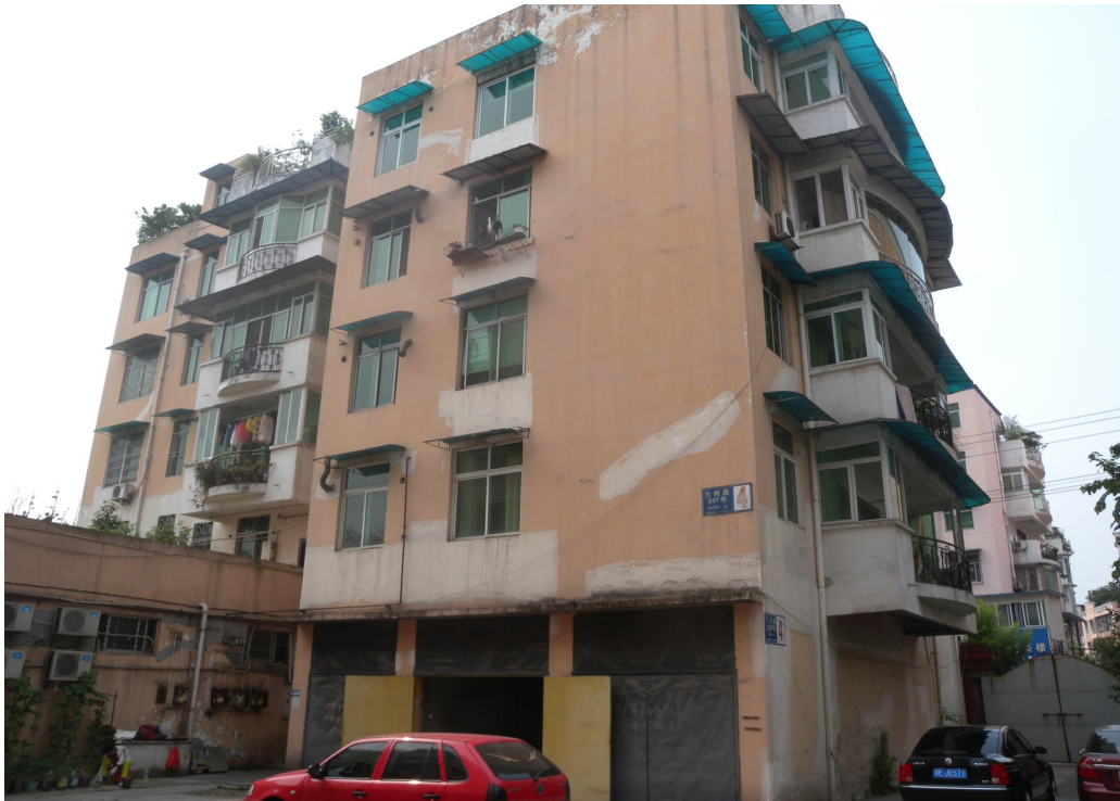
Fig. (14). One bottom frame structure in Wenchuan earthquake.
