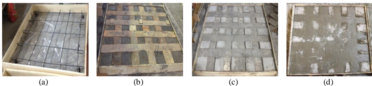
Fig. (4). Specimen fabrication and strengthening procedure of slab type D: (a) placing steel reinforcement into the slab's mould, (b) pre-devising grooves by placing strip moulds into the tension face of slab before concrete hardening, (c) grooves formed on the tension face after removing the moulds and (d) strengthening by applying HPFRCC to the grooves.
