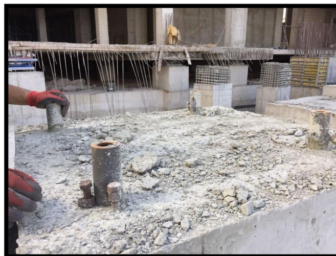
Fig. (13). Isolator's bottom dowels and assistant bolts.
