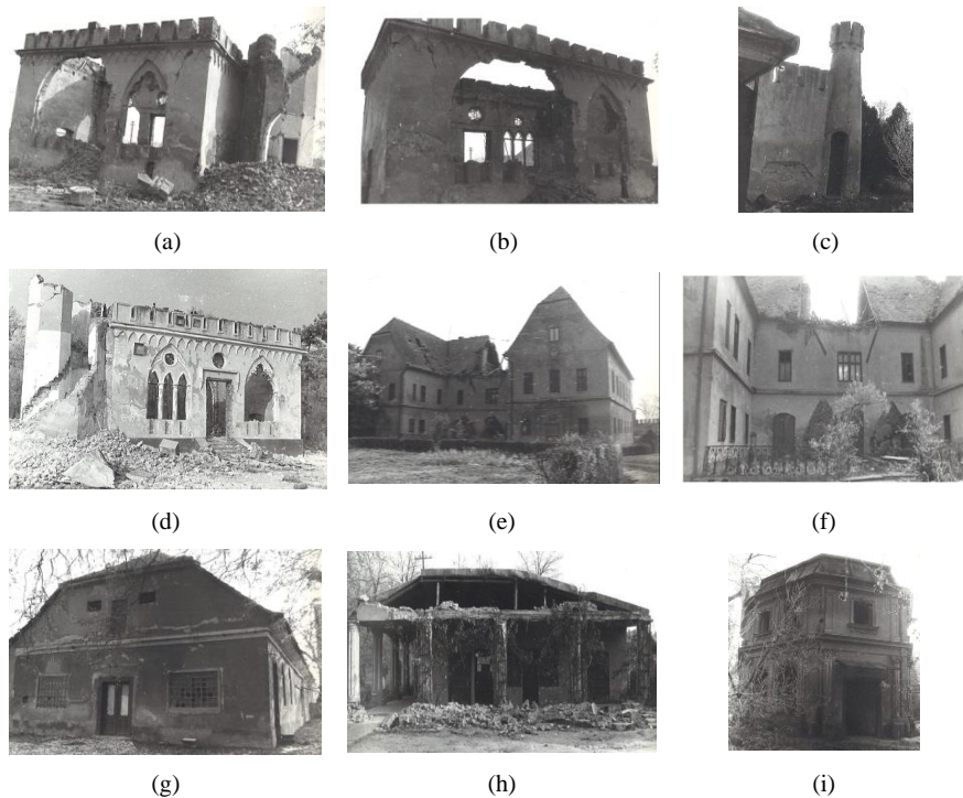
Fig. (2). Post-earthquake damages and failures recorded in the epicentral area near Timisoara after 1991 earthquakes [12].
