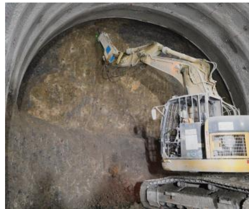
Fig. (7). Irradiation of the tunnel face in contact with the drill tip.
