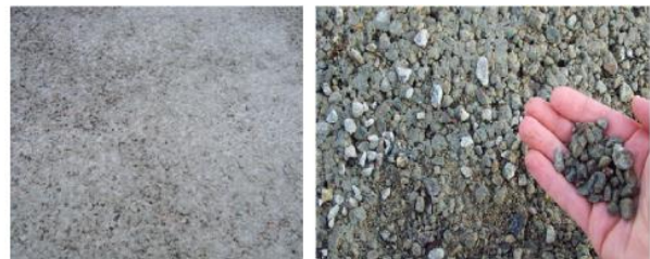
Fig. (1). Clogging and Raveling observed in PC Pavements [5, 25].
