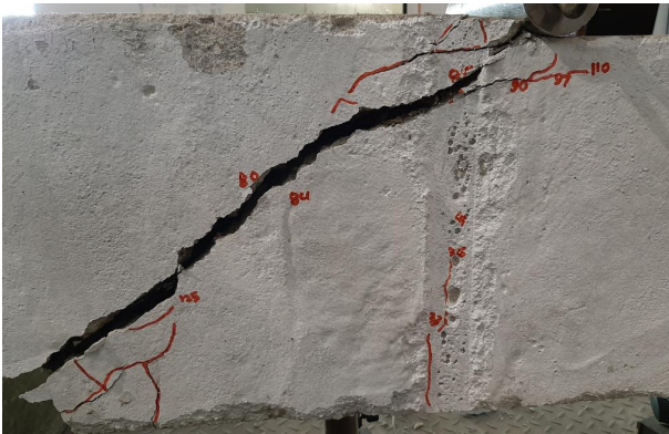
Fig. (20). Enlarge section of the crack.
