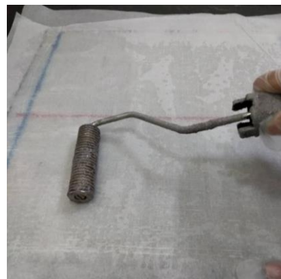
Fig. (4). Rolled the wet GFRP sheet to removed excess epoxy resin and trapped air bubbles.
