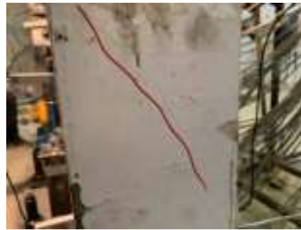
b) Concrete cracks
