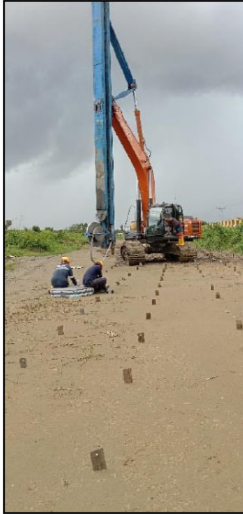
Fig. (2). PVDs installation in Batang Saribas, Betong Division, Sarawak, Malaysia. Note: The sand layer covers the peat, which is part of a drainage system.
