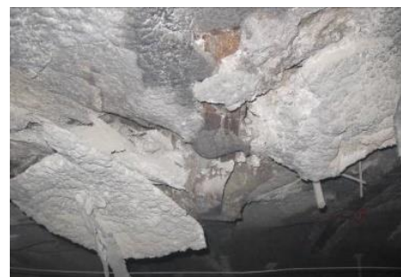
(c) Cracking and spalling of initial support concrete
