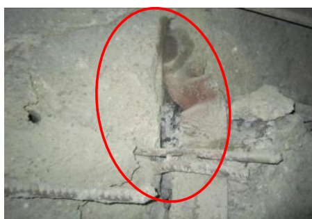
(b) Distortion of the grid steel frame
