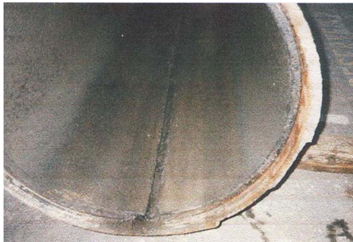
Fig. (2). The groove developed at the invert of the force main in Vancouver [16].
