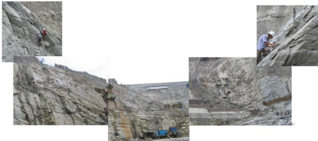
Fig. (11). Dip-angles of unloading fractures varied with the excavation surface of dam base.
