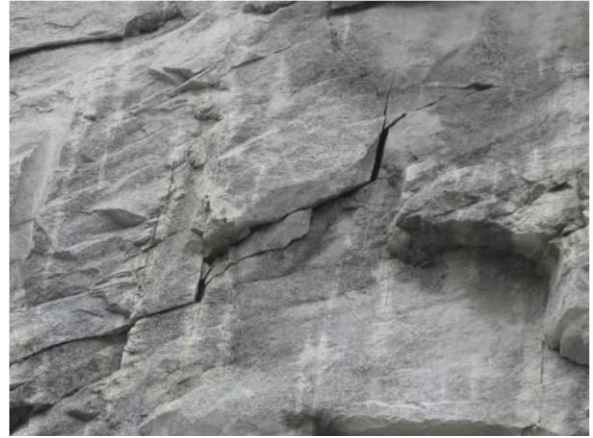
Fig. (7). Shearing along low-dip angle crack and tension along steep-angle crack.
