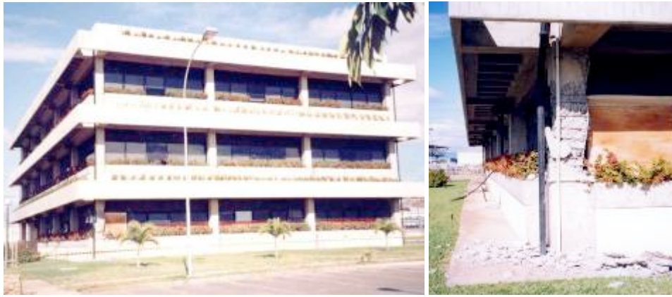
Fig. (6). Effect of short column generated by walls of reinforced concrete. (Photo courtesy of A.Urich).
