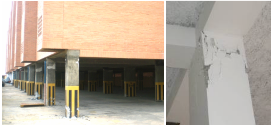
Fig. (7). Story “weak” or “soft” because open space on that first floor. (Photo courtesy of A.Urich).
