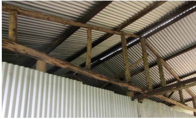
Fig. (9). Timber roof truss forming squares instead of triangles and without longitudinal bracing to prevent the truss from tipping which will drag the other trusses. Source: [36].
