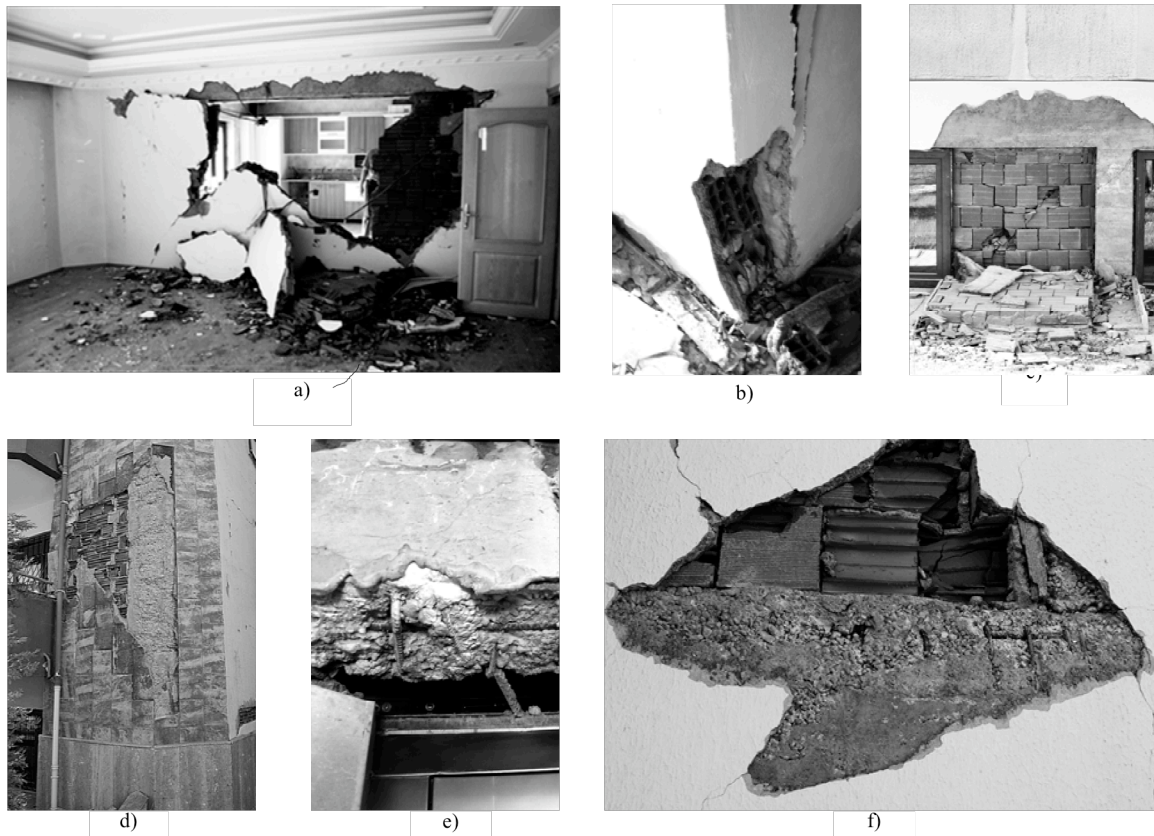
Fig. (3). Observed building damage.
