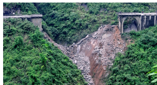
(c) Hong Ni Shi bridge damaged in 2010
