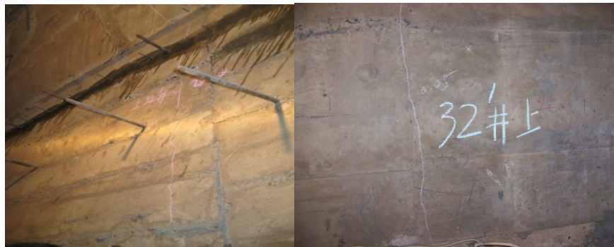
(a) Concrete cracks for arch ring
