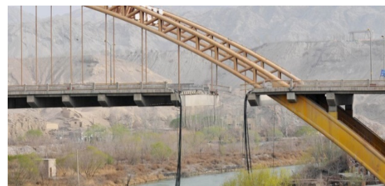
(b) Kong Que He bridge damaged in 2011
