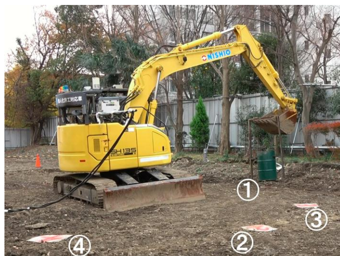
Fig. (8). Image of the worksite. The numbers indicate the mat numbers. The drum is initially placed on mat 1.
