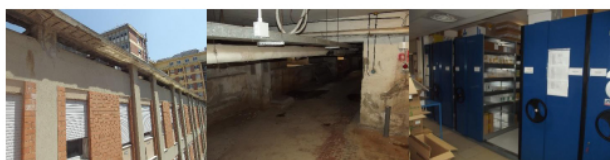
Fig. (25). Examples of degradation of concrete elements (left) and inadequate anchorage of plant systems (centre) and shelves (right) in [HB] building.
