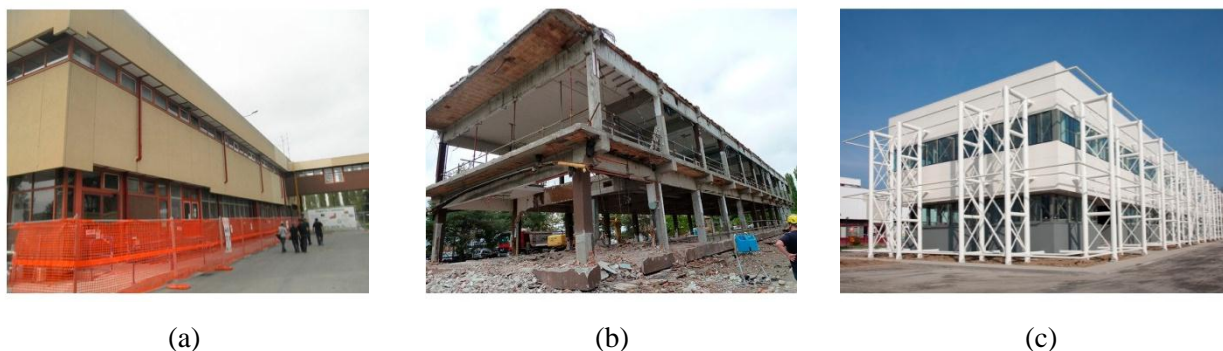
Fig. (1). Sequential steps for the retrofit of an existing RC building: (a) pre, (b) during and (c) post intervention (figures reproduced from [14] under the terms and conditions of the Creative Commons Attribution (CC BY) license).
