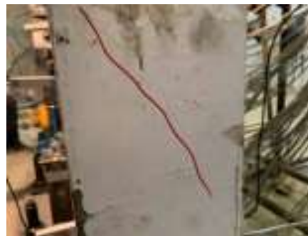
b) Concrete cracks
