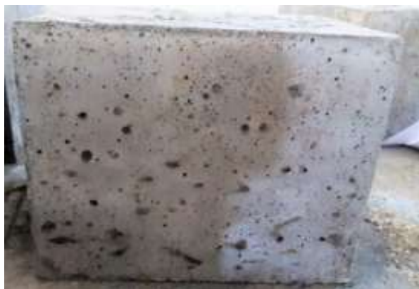
Fig. (5). Bug holes found on concrete surface (75% silica sand non-magnetic water).
