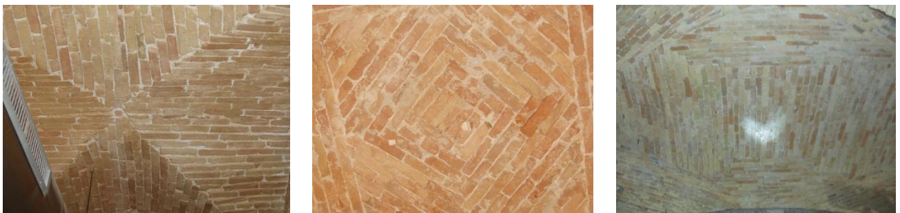
Fig. (5). Different textures of masonry vaults in the downtown of Cagliari (courtesy of Prof Cazzani, University of Cagliari, Italy).
