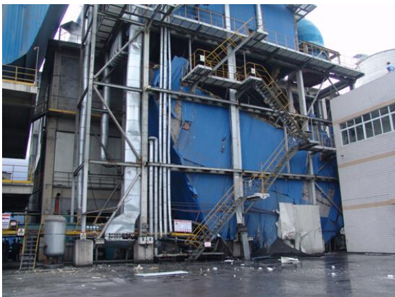
Fig. (3). Collapse of dust-settling compartment.
