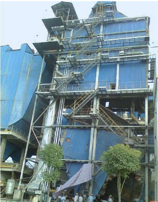
Fig. (2). The main scene of the accident.
