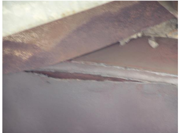
Fig. (5). Tearing seam between the attachment weld.
