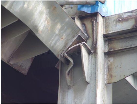
Fig. (7). Damage of beam-column joint.
