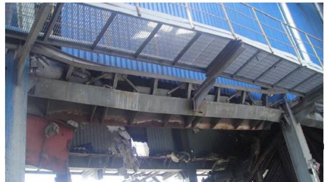
Fig. (6). Distortion of bearing beam.
