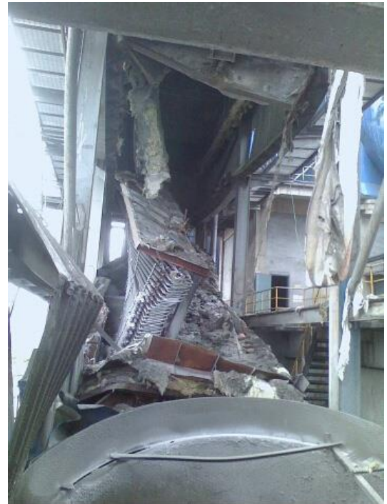
Fig. (4). Collapse of super-heater tube chamber.
